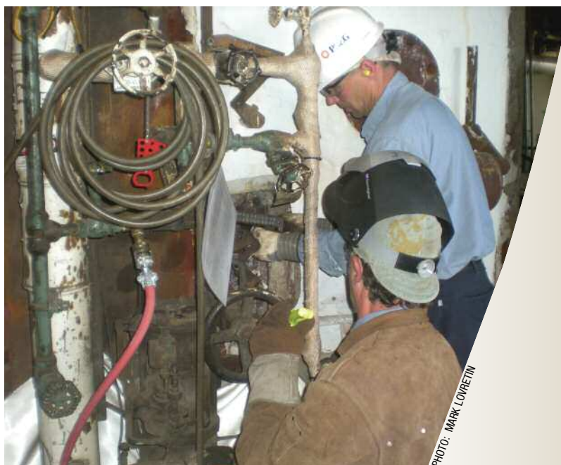
The Sewaren generating station marked 60 years of service last November.
