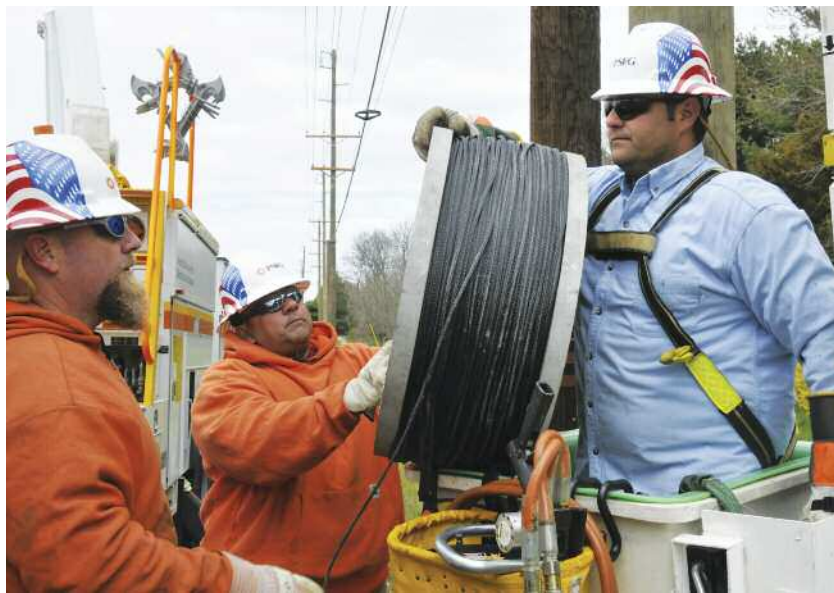
From left: Linemen Scott McLain, Tony Russo and Shane Greening from the Mobile Construction Workforce-North Zone prepare for the installation of a new 69kV circuit in Hillsborough, N.J.
